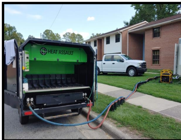
Figure 4. Heated glycol being pumped into Heat Assault radiators inside the apartment (Dini Miller Virginia Cooperative Extension)
