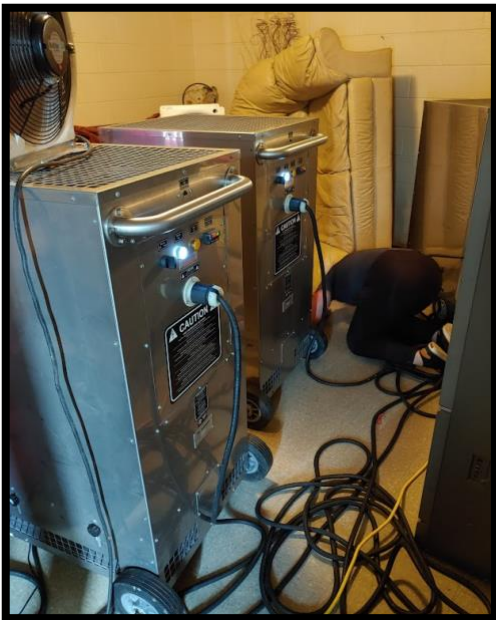
Figure 6. Setting up the TempAir system equipment in preparation for heat treatment (Dini Miller Virginia Cooperative Extension).
