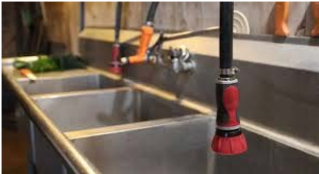
Figure 1: Stainless steel vegetable wash station (provided by the UVM Ag Engineering)
